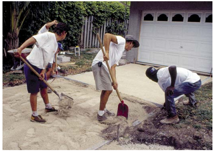
More efficient bedding sand distribution, screeding tools and methods can reduce crew members from four shown here to one or two persons. The result is increased productivity through saved labor hours.
