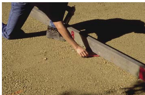
Figure 1. All effort placed into making a smooth base surface will result in a smooth paver surface. The base surface is checked with a straightedge after compaction.
