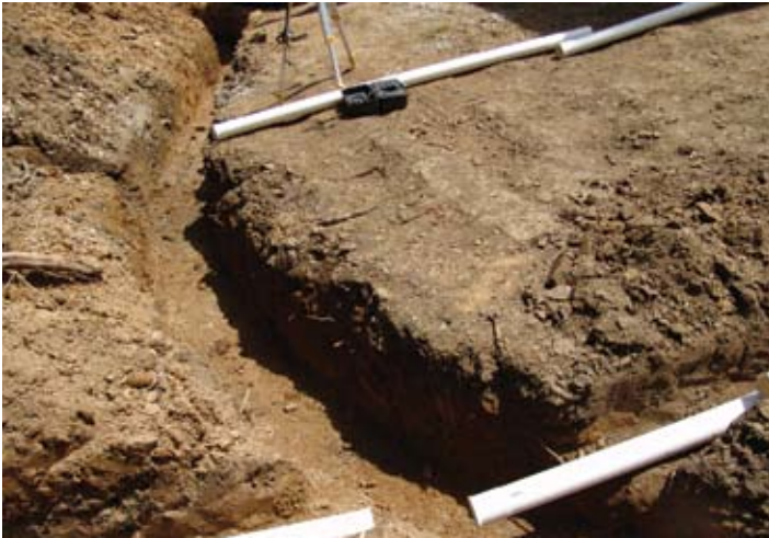
Figure 1. Raised patio construction begins with excavating trenches for footers prior to lining them with geotextile and filling them with compacted, dense-graded aggregate. For this project the footer depth was a generous 3 ft (0.9 m). PVC pipe is readied for down-spout drainage.
