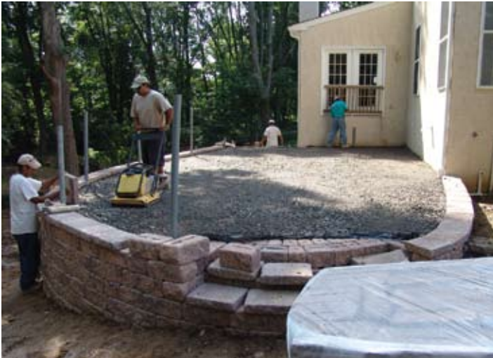
Figure 5. Placing and compacting a 4 in. (100 mm) thick base layer provides a medium to enhance the sloped surface for drainage.
