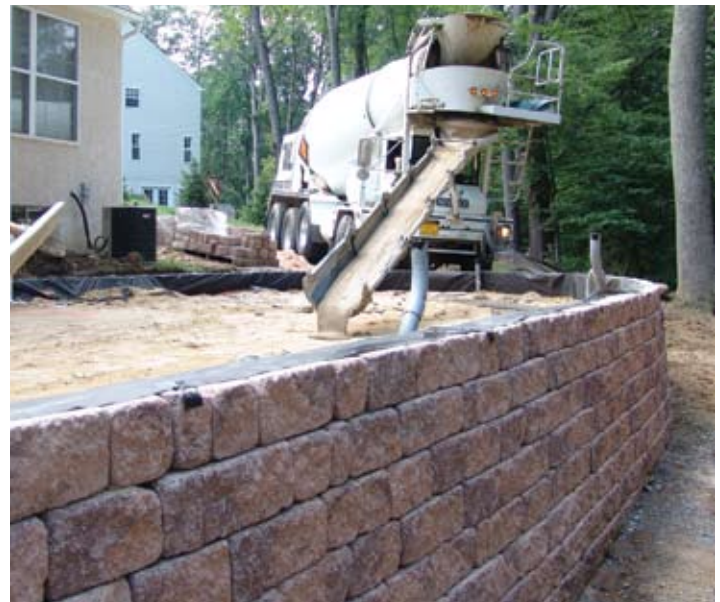
Figure 4. The final (fourth) pour with conduit for wiring sprouting well above the surface with tops taped shut.
