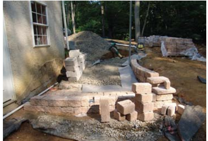
Figure 2. At a minimum, the first course of retaining wall must be completely submerged within the ground. Retaining wall blocks must be at the correct elevation and be plumb before placing higher courses. All wall units in this project were glued with adhesive. Note the geotextile flaps emerging from under the footer and that the white PVC pipe for drains or can sleeve supply pipes.
