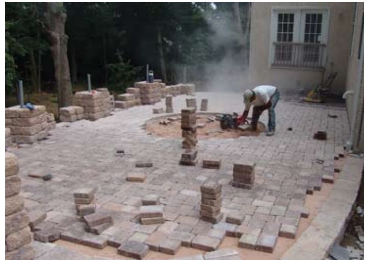
Figure 6. Once the bedding sand is placed and screeded, pavers are installed, cut, compacted, joints filled with sand and the area compacted again just like any at-grade patio project. Note the columns rising to accommodate fencing.
