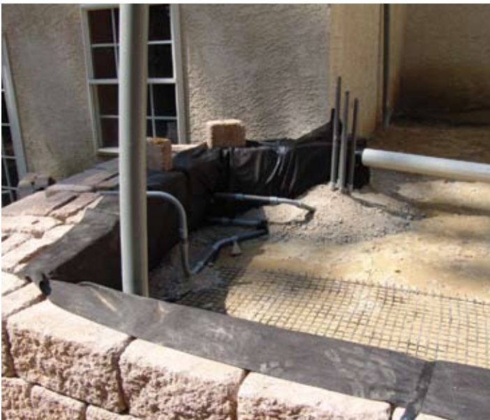
Figure 3. Each flowable fill pour is 18 in. (450 mm) deep and its pancake batter consistency fills around drainpipes and conduit.
