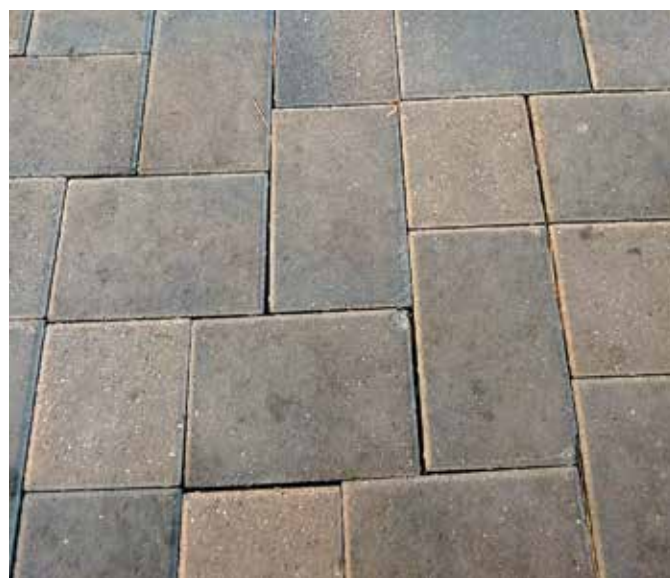
Figure 20. Variation in the joint width is a typical present in ICP with excessive joint width.
