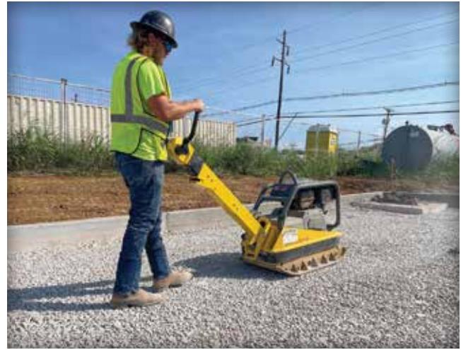
Figure 21. A larger reversible plate compactor is used to compact ASTM No. 57 stone base.
