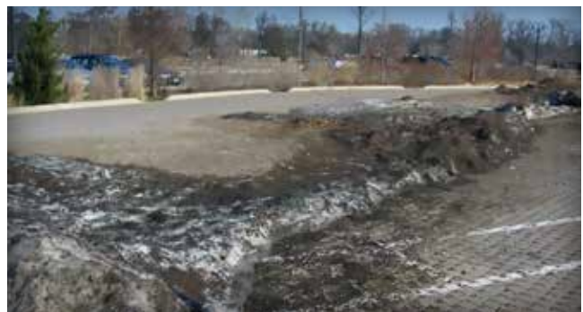
Figure 26. This is an example of snow that should have been deposited on a grassy area. If such areas are not available, then vacuum clean the PICP in the early spring.
