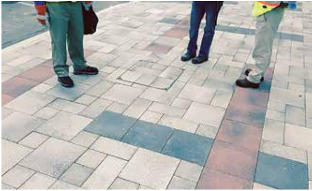
Figure 27. Example of a utility cover that does not fit neatly into the paving pattern.
