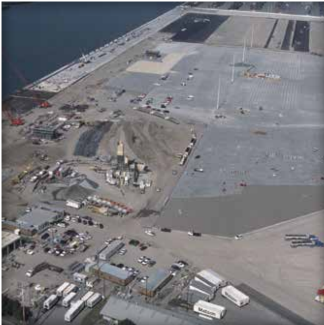
Figure 14. The Port of Oakland, California, is the largest mechanically installed project in the western hemisphere at 4.7 million sf (470,000 m 2 ).
