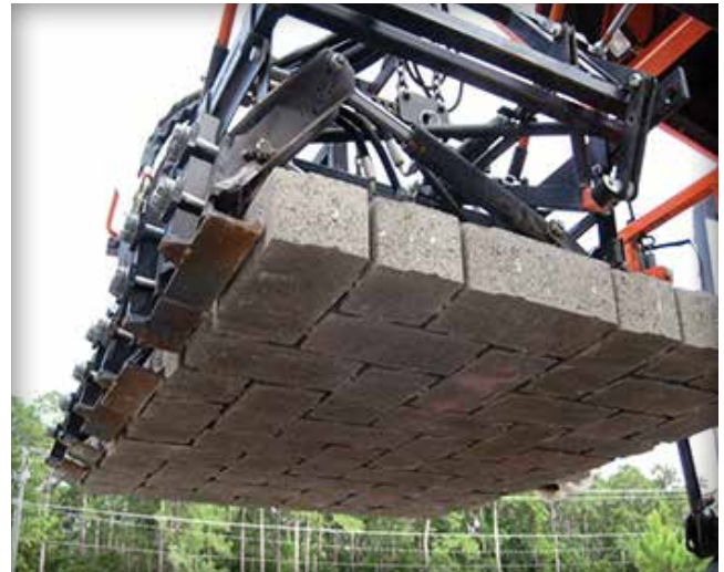
Figure 3. A cluster of pavers (or layer) is grabbed for placement by mechanical installation equipment. The pavers within the cluster are arranged in the final laying pattern as shown under the equipment.
