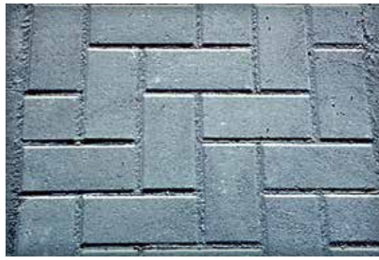
Figure 6. A close-up of the concrete paver surface at the PTI test track.
