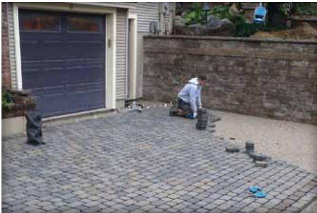
Figure 11. Concrete pavers installed to accommodate permeable bedding and jointing materials, all supported by a permeable stone base.
