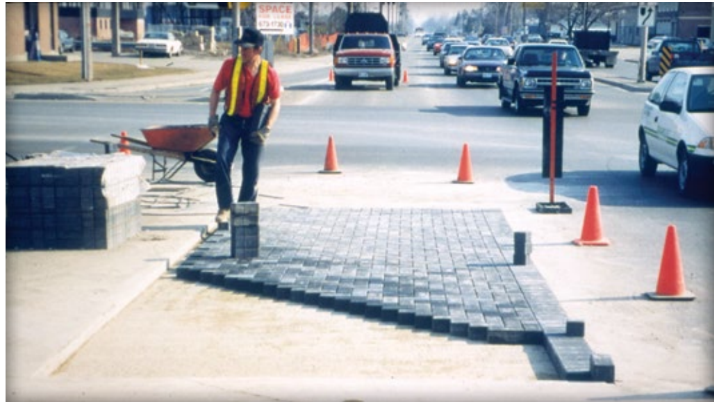
Figure 12. Pavers are laid in a 90 degree herringbone pattern between the border courses.
