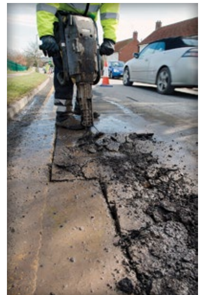
Figure 1. Repairs to utilities are a common sight in cities, incurring costs to cities and taxpayers.
