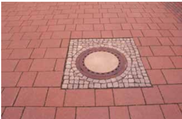
Figure 29. Filling the outside of a utility cover with mortar-set stone paving units
