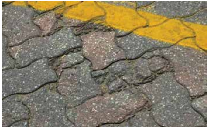
Figure 17. Damaged pavers can be caused by excessive movement of the base or excessive concentrated loads applied to the surface.
