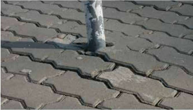
Figure 22. Heave is typically seen near structures that have moved due to freeze-thaw action.
