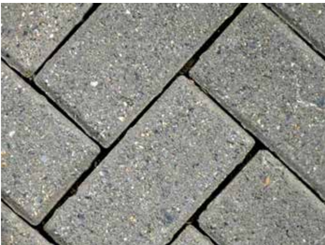
Figure 24. Joint sand loss should be repaired when the void created is greater than 1/2 in. (12 mm).
