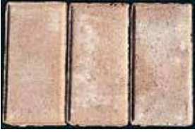
Pavers with efflorescence
