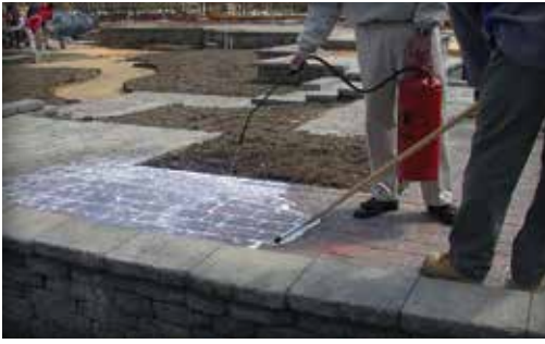
Figure 3. This liquid joint sand stabilizer is applied with a low-pressure sprayer and squeegeed across the surface after allowing some time for soaking into the joints. This helps maintain slip and skid resistance of the paver surface.
