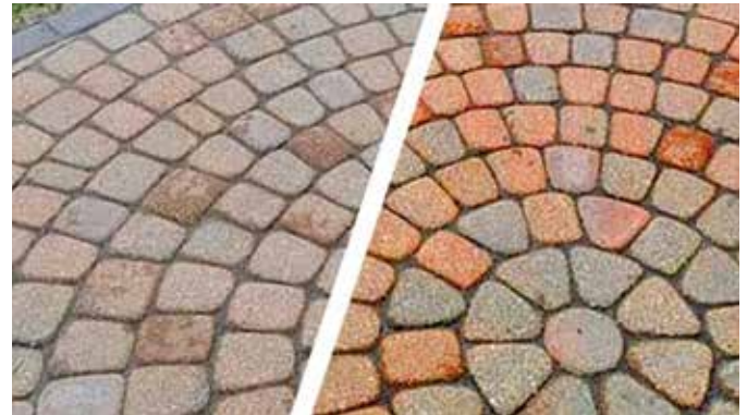
Figure 14. Cleaning the ICP surface can remove fine particles lodged in the pores of the concrete surface to rejuvenate the color.
