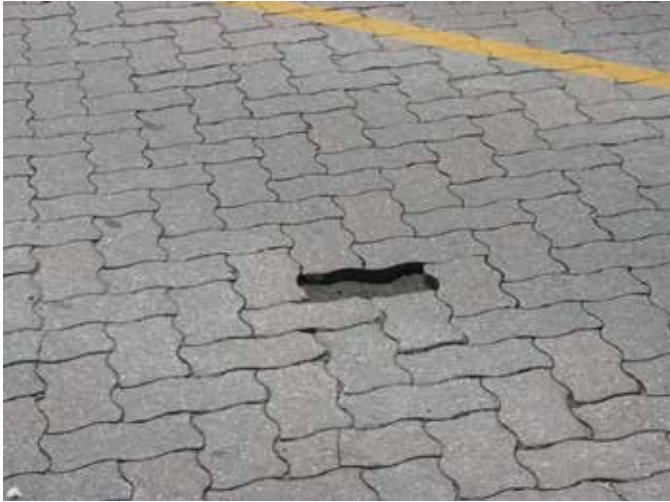
Figure 25. Missing pavers should be replaced as soon as possible to avoid damage to the surrounding units.
