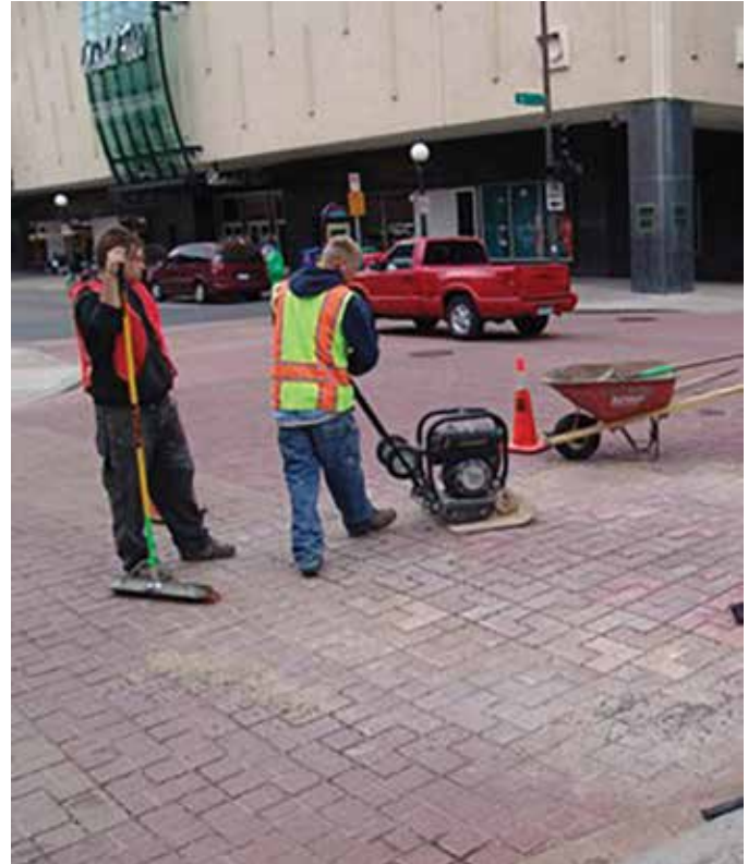
Figure 42. Pavers are compacted into the loose bedding sand. Joint sand is then swept and vibrated into the joints until they are filled to complete the repair.
