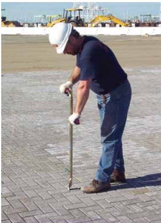
Figure 41. An alignment bar and string line can be useful to tweak the pattern and make it line up with the surrounding undisturbed paver.
