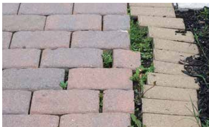
Figure 19. Lack of an effective edge restraint has allowed the pavers to separate and compromise the structural capacity of the ICP.
