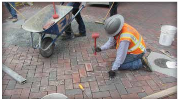
Figure 5. The final paver is inserted, the reinstated area compacted, joints filled, and compacted again. There are not cuts or damage to the pavement surface.
