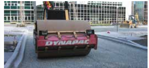
Aggregate base and subbase are spread and compacted; pavers are delivered ready to install. After placement, joints and/or openings are filled with small aggregate. Then pavers are compacted.
