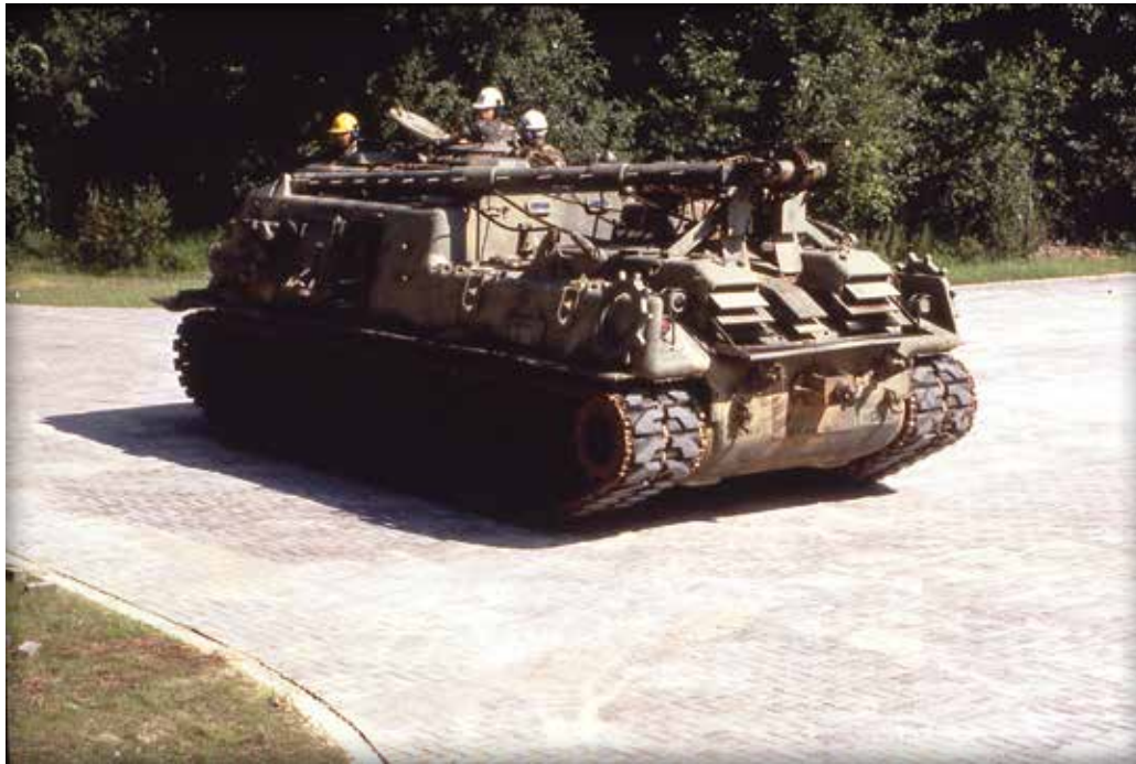
Figure 13. The completed paved area from Figure 12 receives tank traffic at the U.S. Army Proving Grounds in Aberdeen, Maryland.
