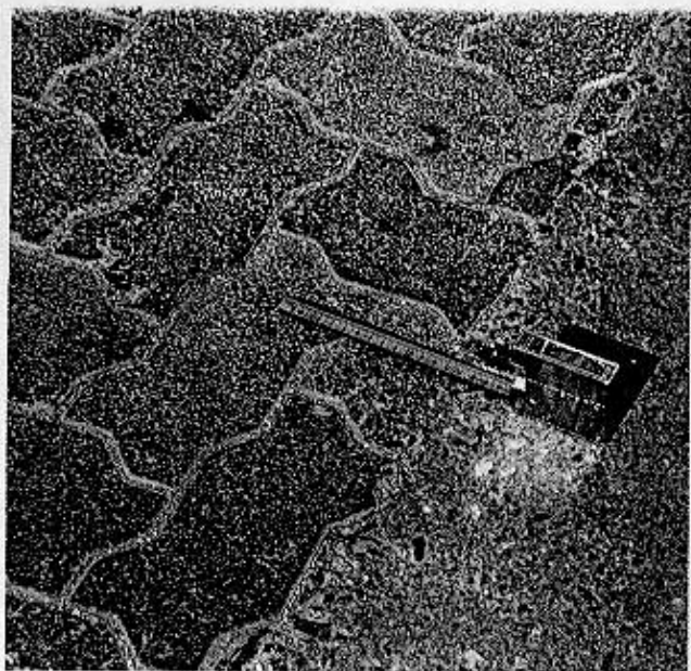
Figure 7. Close-up photograph of a successful joint solution between interlocking blocks and the existing asphalt surface.
