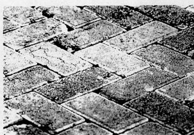
Figure (3) Photograph showing typical defects
