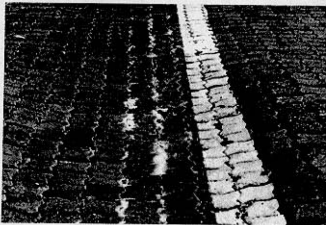
Figure (2) Photograph showing severe deflection in pavement.
